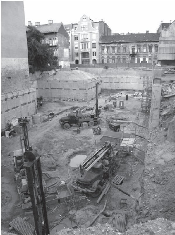
Figure 8. Budapest (Hungary), construction works on the site of demolished 19th-century dwelling houses just behind the great synagogues of the town centre (Photo: Pál Lóvei).
