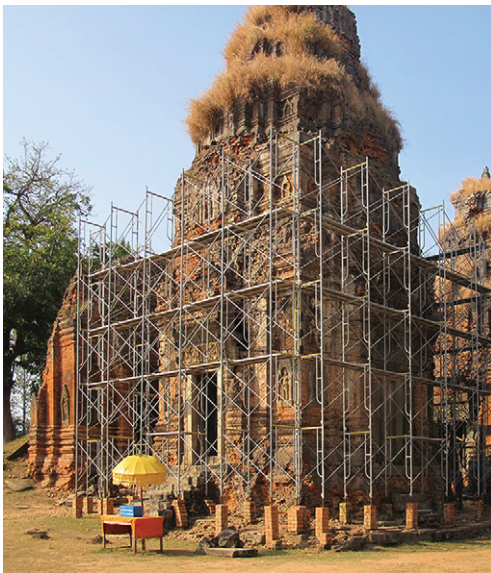
Conservation work in progress on one of the brick-built sanctuary towers at the late ninth-century temple of Lolei, south-east of Angkor.
