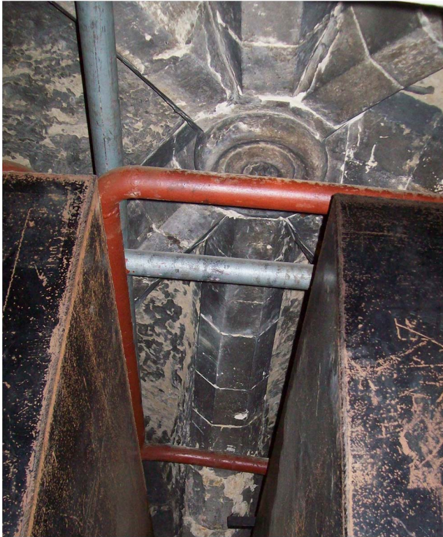
Fig 9. The seven-ribbed vault over the main space of the crypt of the Lincoln Cathedral treasure house, slightly obscured by modern pipework. Photograph: © author
