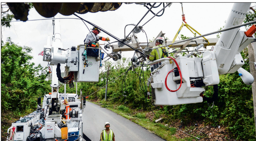
Transmission and distribution specialists assigned to Company D, 249th Engineer Battalion (Prime Power) of the US Army Corps of Engineers, repair power lines in Rio Grande, Puerto Rico, after Hurricane Maria. Photo credit: Master Sgt. Joshua L. DeMotts, US Department of Defense.
