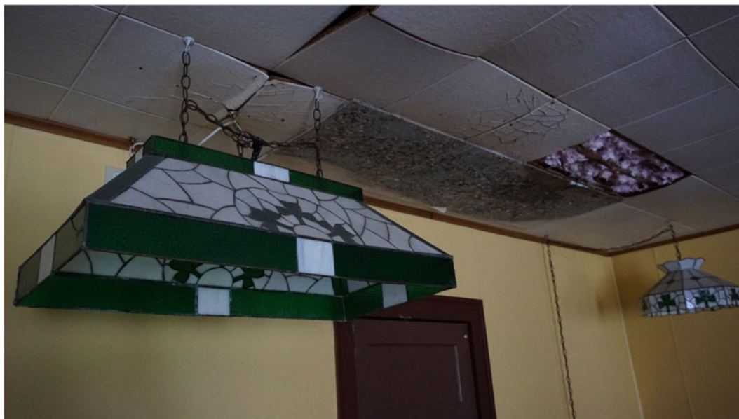
Figure 4. The crumbling ceiling of a resort in 2019. Photo by author.
