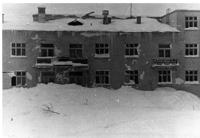
Fig. 14. Avalanche deposits in front of Sakhalin sanatorium; the ground floor is completely under snow (12 January 1965; photograph from archives of Sakhalin UGMS).
