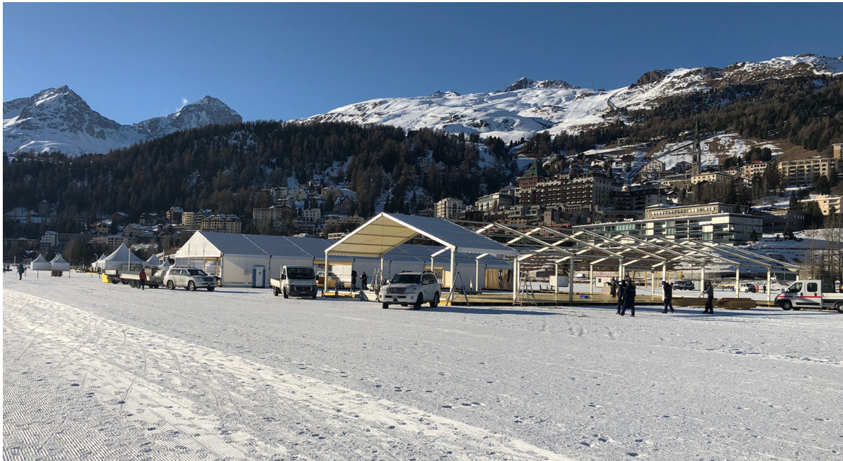
Fig. 1. Building up of a 130 000 m 2 tented village on Lake St. Moritz (Switzerland). At the date of the photo (17 January 2022) the ice was about 45 cm thick and was covered by a layer of about 4 cm of groomed snow.
