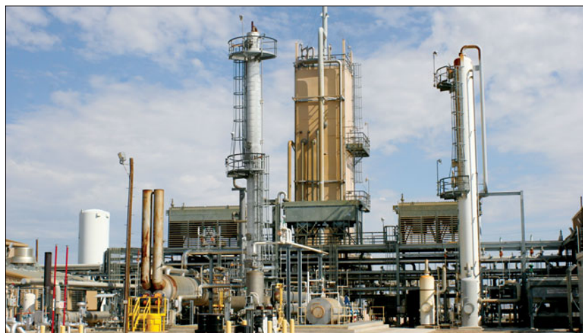
US Bureau of Land Management’s crude helium enrichment facility near Amarillo, Texas.
