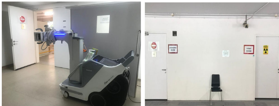
Radiology Facilities in the Flu Screening Area (FSA).
