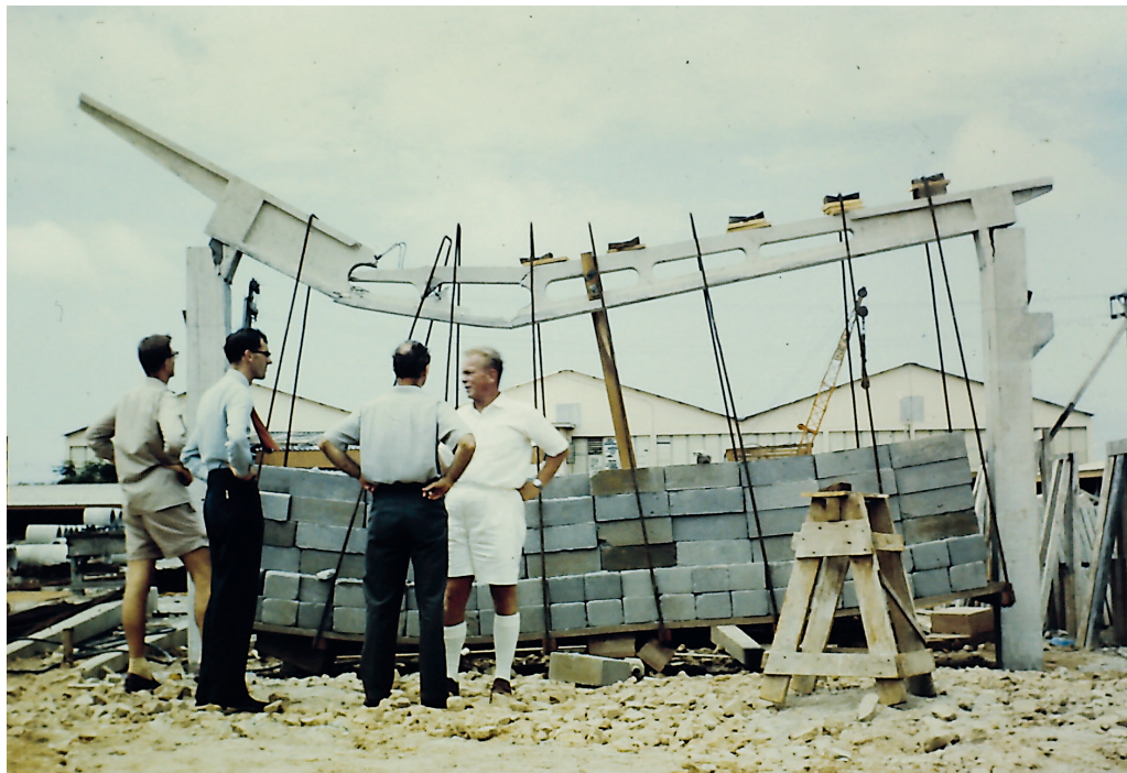
Fig. 18. Tema Community 1 , stress test on the roof beam of the Outpatients Department, photograph of 1958 by Michael Hirst
