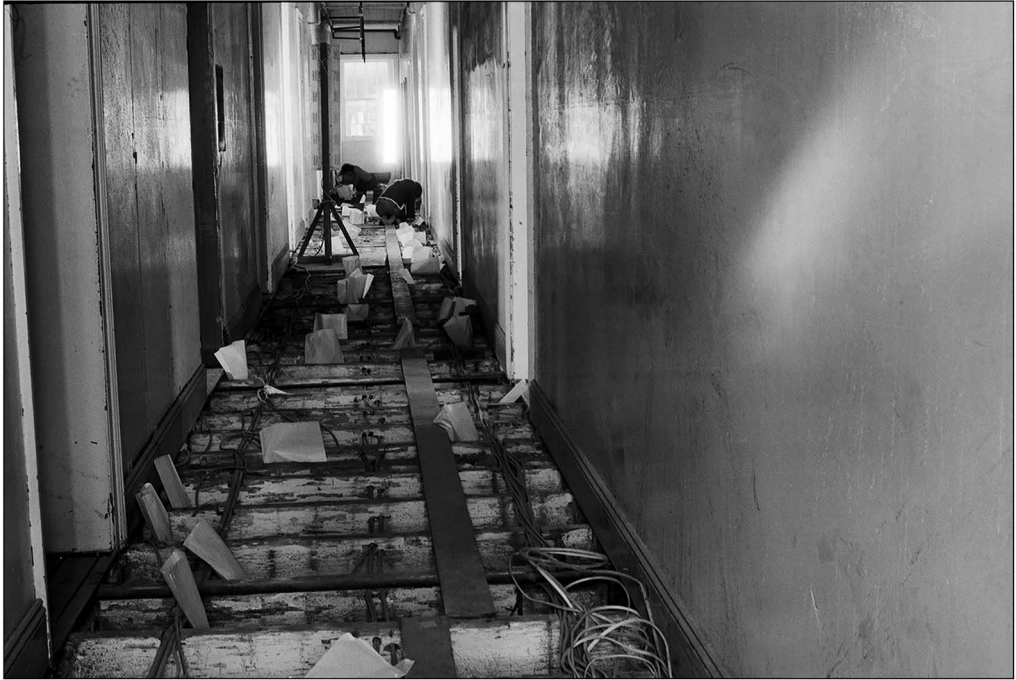
Figure 3. Excavation of the underfloor deposits in 1980–1981 showing the system of joists beneath the floorboards (photograph courtesy of Hyde Park Barracks Collection, Museums of History NSW).
