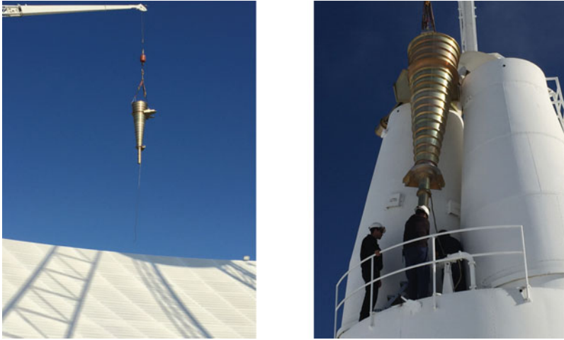
Figure 1. Installation of the new wideband feed on 2015 August 21. ( Left ) New 1.4–1.9 GHz feed being lifted onto the 70 m DSS-43 antenna at the Canberra Deep Space Communications Complex. ( Right ) Installation of the new feed into the Cassegrain focus “cone” of DSS-43. The scale of the new feed is evident by comparison with the individuals in the image.
