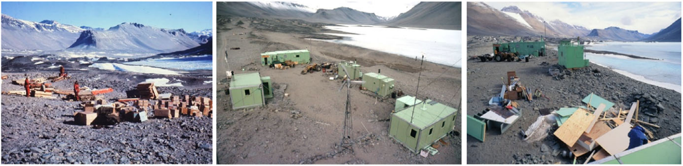
Figure 3. Left – Vanda Station under construction in 1968. Centre – Vanda Station in operation. Right – deconstruction underway in 1993. Note the gradual encroachment of the lake up to the station site (Images Antarctica New Zealand; A.D.A.M.).
